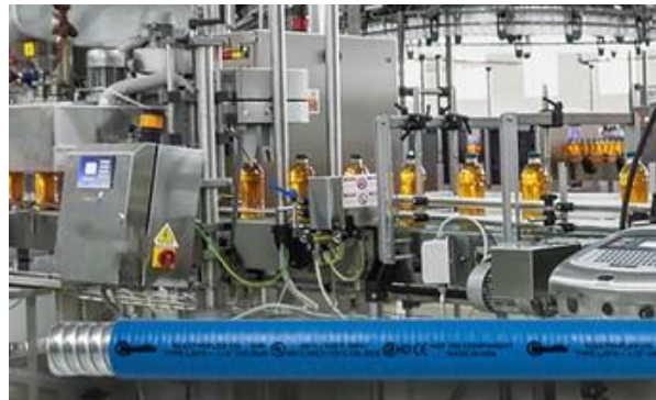
Figure 1. Modern industrial food processing involves miles of electrical wiring, which must be safely routed within flexible conduit raceways. Source: Electri-Flex
